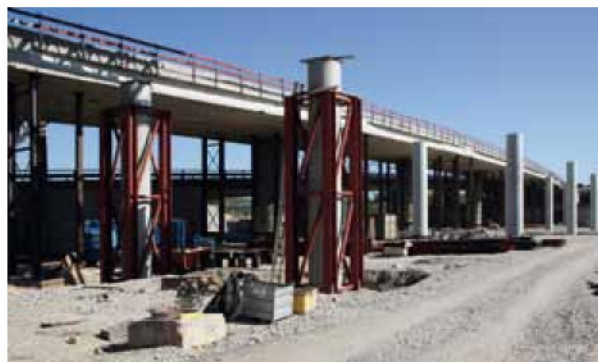
4 Viaduct Freimann at the BABA 9 temporary support for the installation of bridge bearings © Maurer Söhne GmbH & Co. KG
