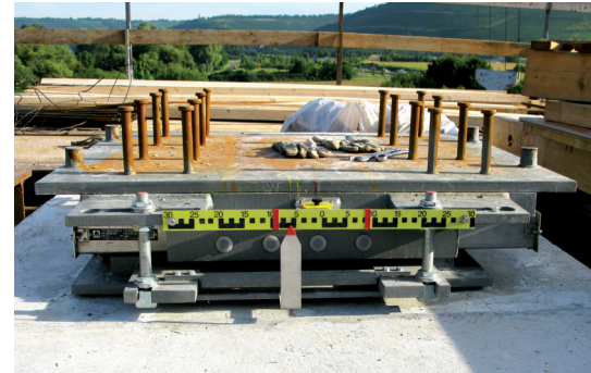
Installation of an MSM Spherical Bearing on a pier head. To be followed by the superstructure in a free cantilever construction method. At the front side the fixation elements can be discerned.
