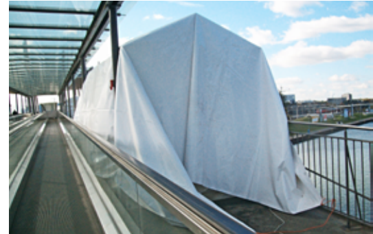
For aesthetic reasons, the installation of the dampers had to be carried out underneath a tent.
