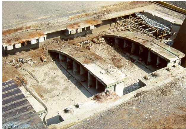
First, the upper plates of the old roller shutter joint were removed. The loosening of the anchor screws was not possible without destroying those anchor screws
