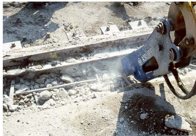
The concreted edge construction had to be chiselled out. At the abutment, the removal of the edge construction was not required.
