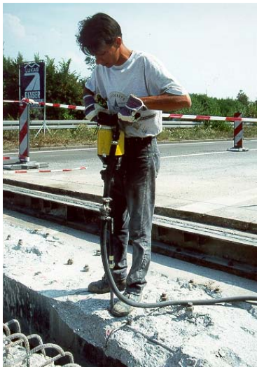
Drilling works for inserting additional reinforcement that anchor the new modular joints.
