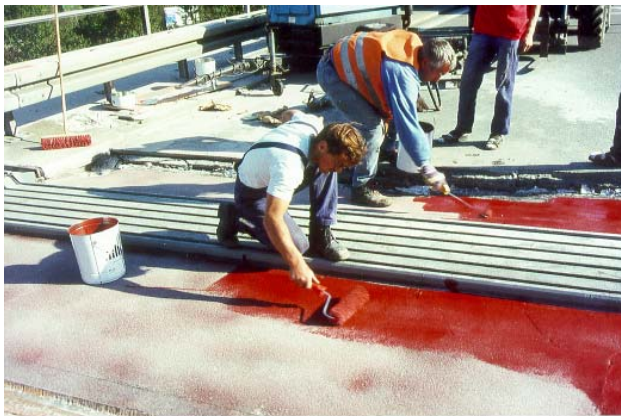
Sealing the cured concrete with epoxy concrete and final application of quartz sand.
