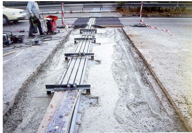
Accelerators for curing were not applied.
