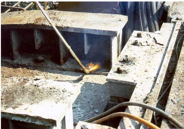
After burning away the respective anchor screws, the sliding guides were removed.
