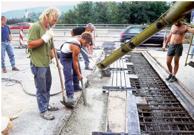
After placing the formwork, concrete of German grade B35 is being applied and cured.
