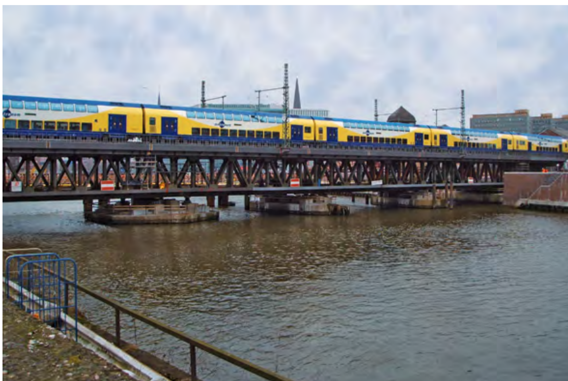
Railway Bridge Oberhafen: Technical challenge were passing trains which caused uplift forces. The problem was solved by way of special uplift spherical bearings.
